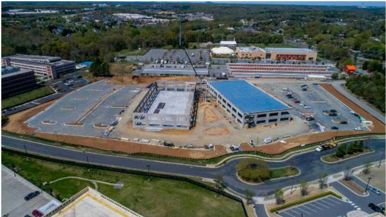
A drone shot of construction at the Edison at Arrowood, a "creative office" building opening this summer. - Courtesy Colliers International
