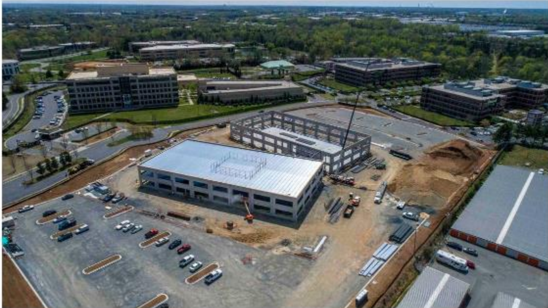
A drone shot of construction at the Edison at Arrowwood, a "creative office" building opening this summer. Courtesy Colliers International
